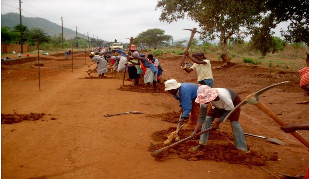
Picture 6: Labour maketh man: Labour intensive methods create jobs and ensure skills transfer to communities
